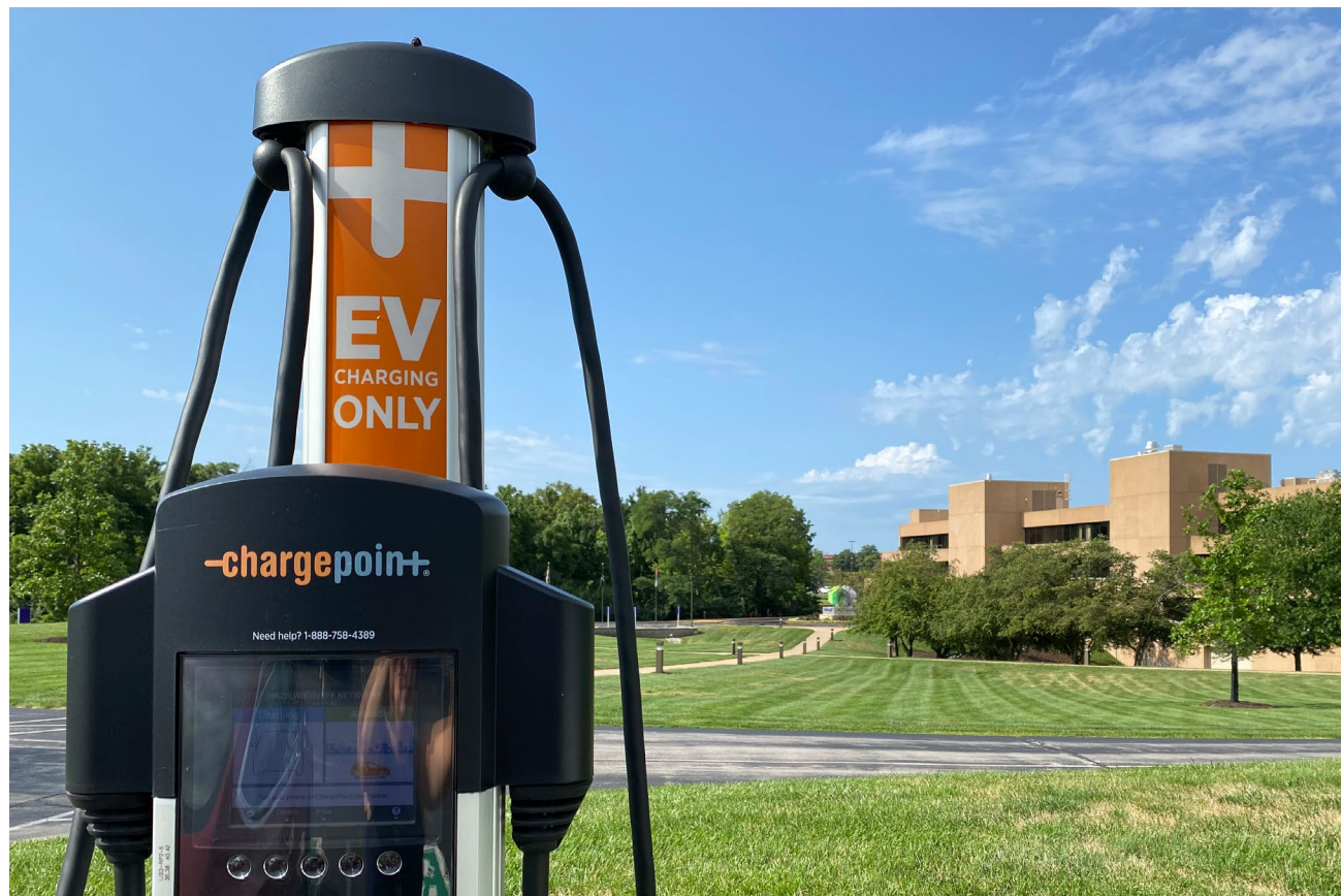
Electric vehicle charging station available for employees
